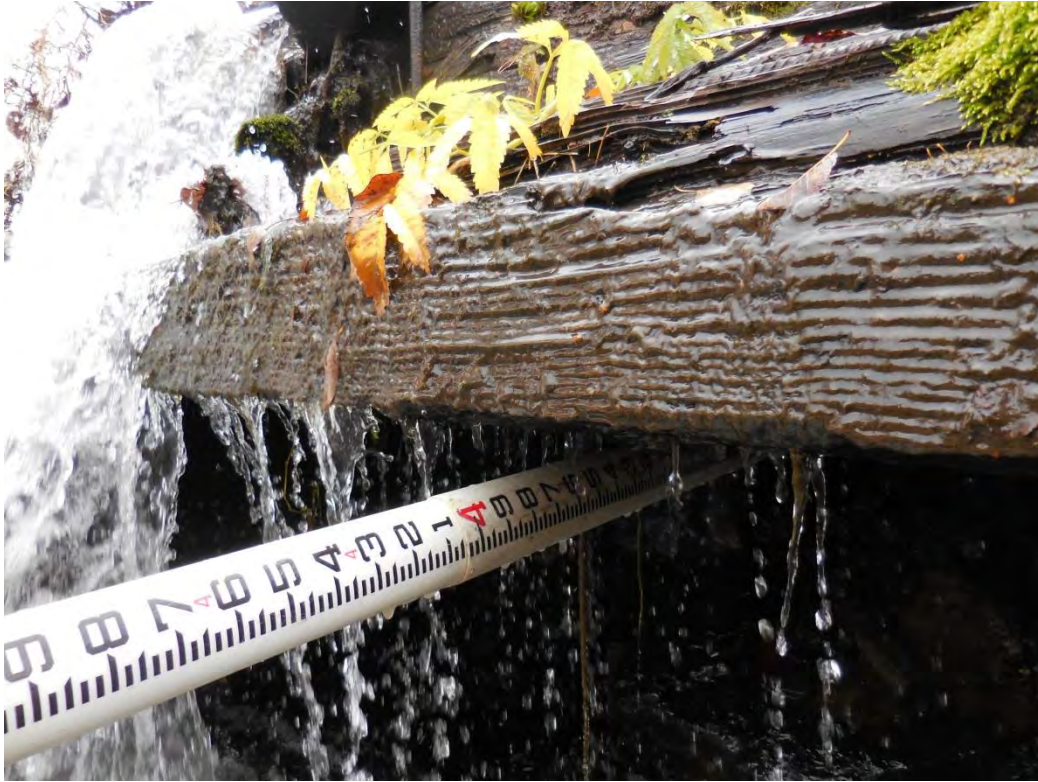
Photo #11 – View of undermined (4') area under Sill #4 at west.
