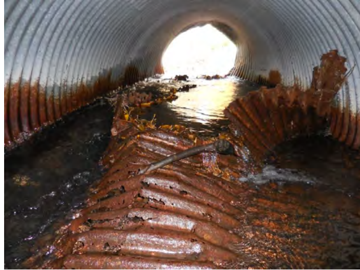
Figure 7: Culvert failure near inlet
