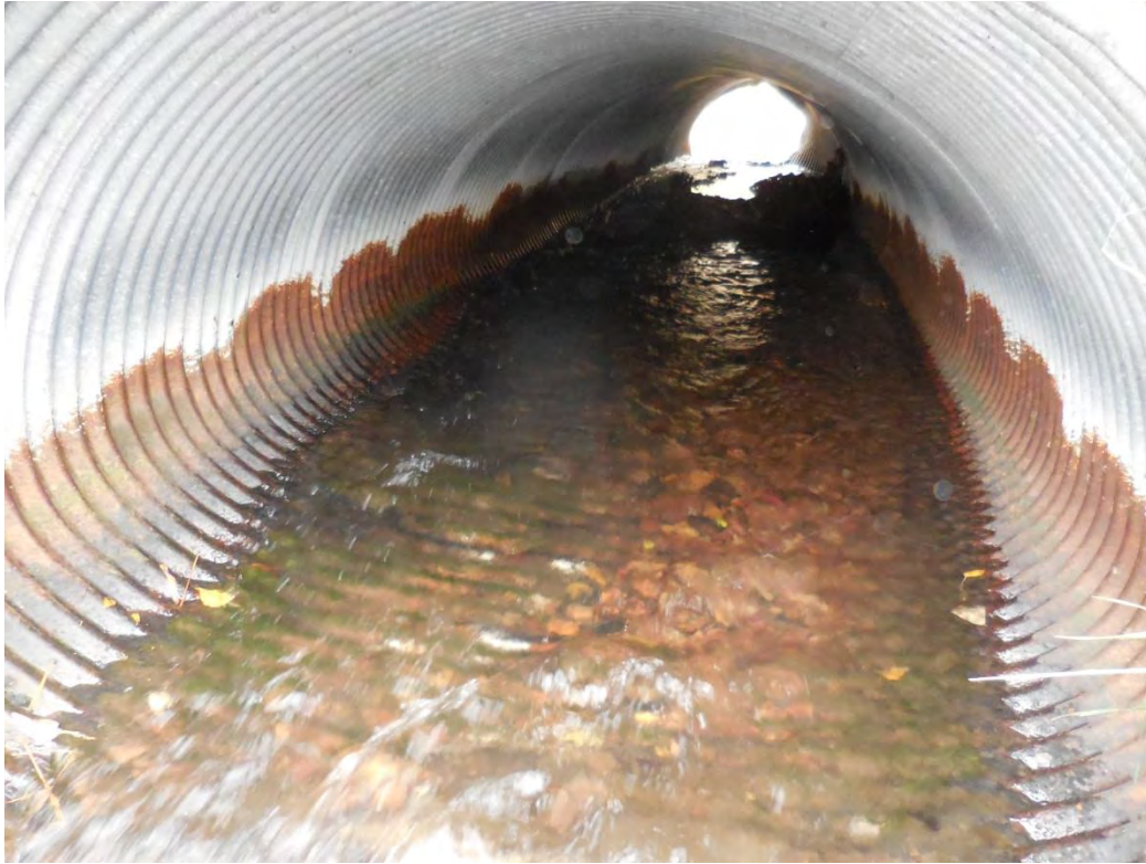
Photo #7 – View of culvert condition near outlet. Note corrosion and deformation.
