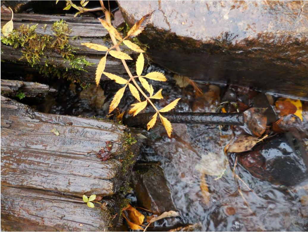
Photo #13 – View of past repair efforts with rebar on wall members, note split and ineffectiveness of rebar.
