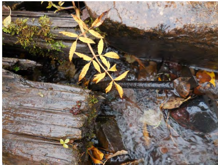
Figure 6: Previously attempted repair has failed
