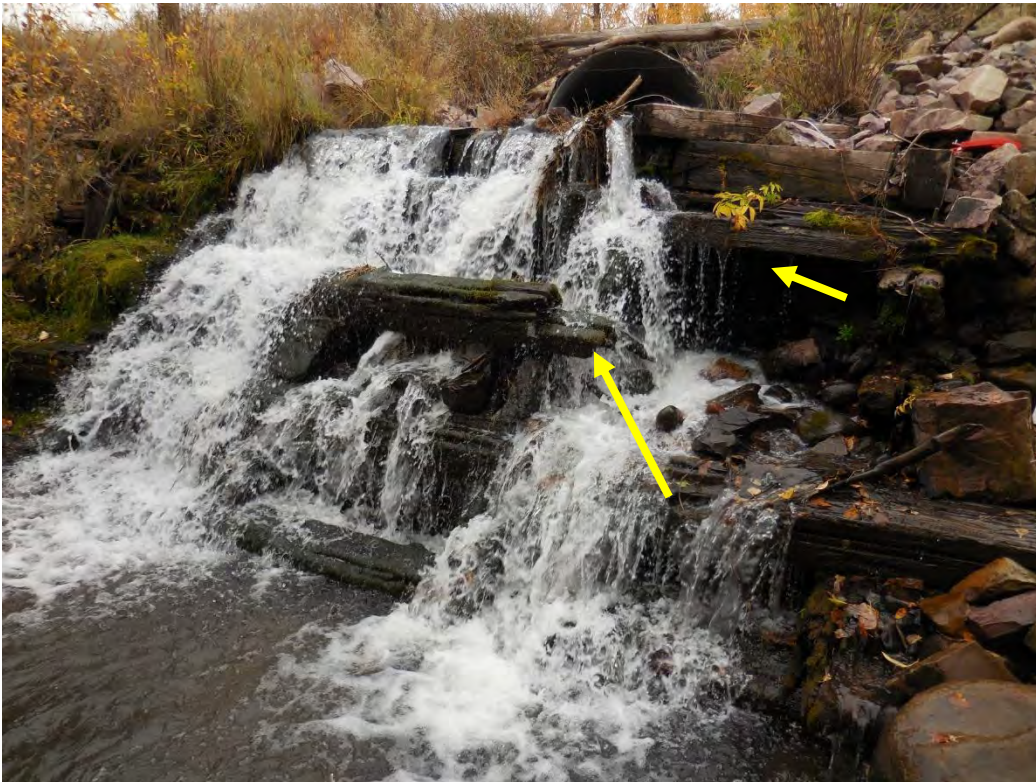
Photo #10 – Another view of timber fish barrier. Note crib member loss at right and area of visible undermining.
