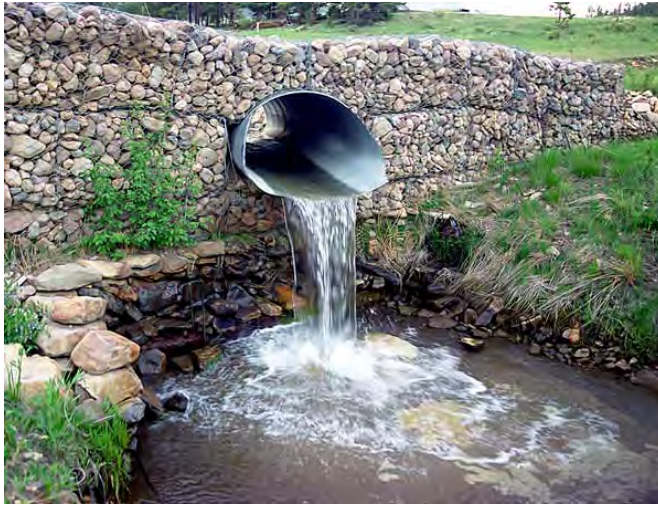
Figure 10: Perched culvert w/gabion retaining wall (Photo courtesy of George Long, Region 3 USDA Forest Service)
