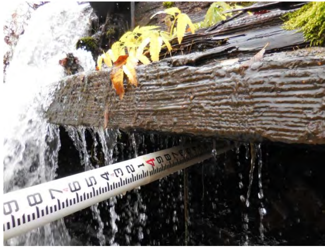
Figure 5: 4' horizontal undermining under Sill #2
