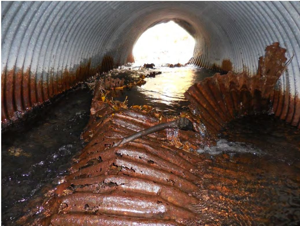
Photo #8 – View of culvert failure approx. 15' from inlet. Note complete section loss and corrosion.
