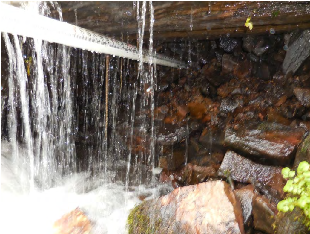
Photo #12 – Another view of undermining under Sill #4.
