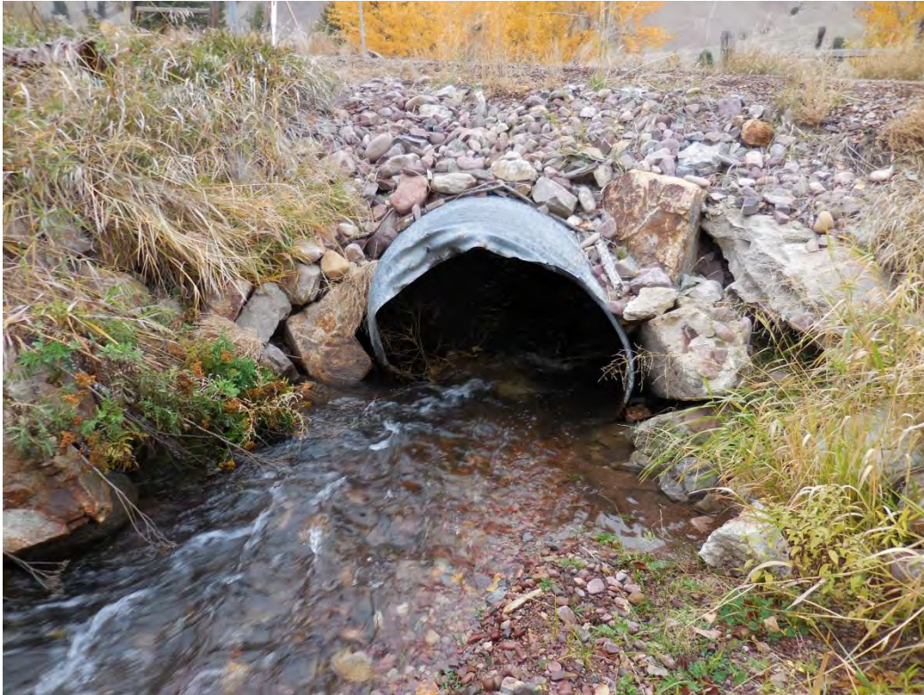
Photo #3 – View of existing culvert inlet, note poor stream alignment and aggradation upstream.
